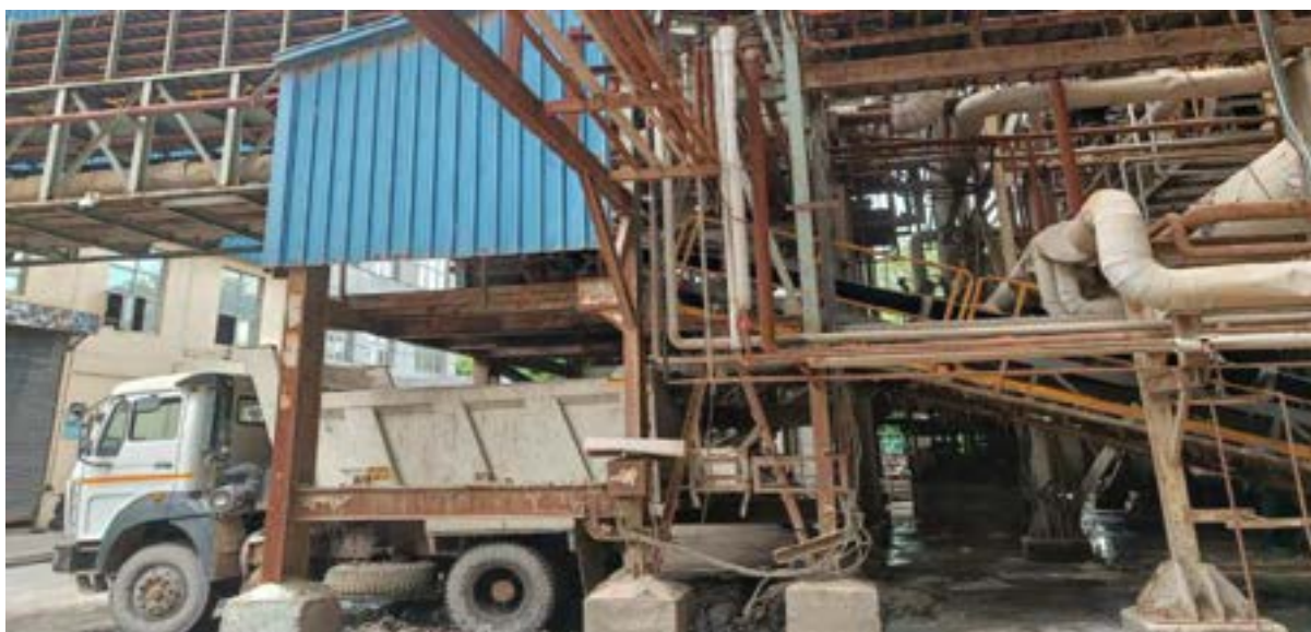
Fig 18: Bottom Ash handling
