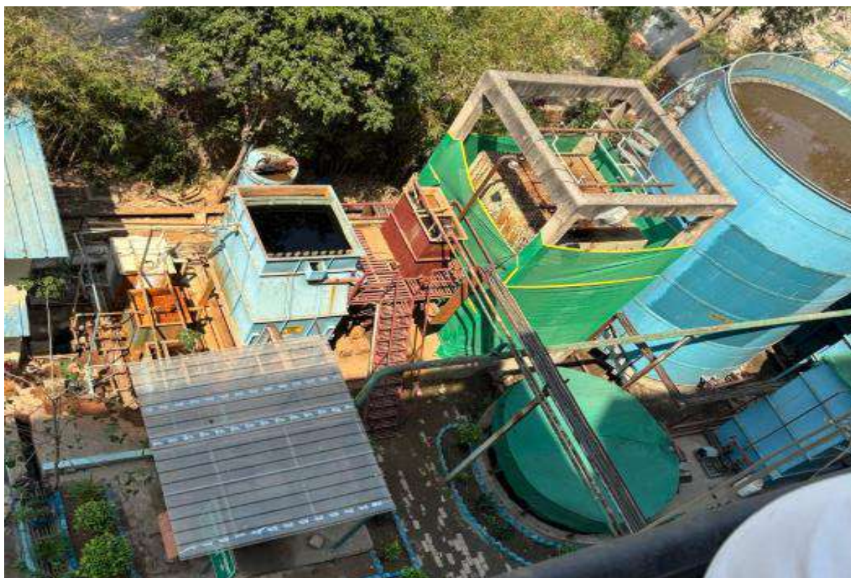
Figure 16: A Leachate Treatment Plant
