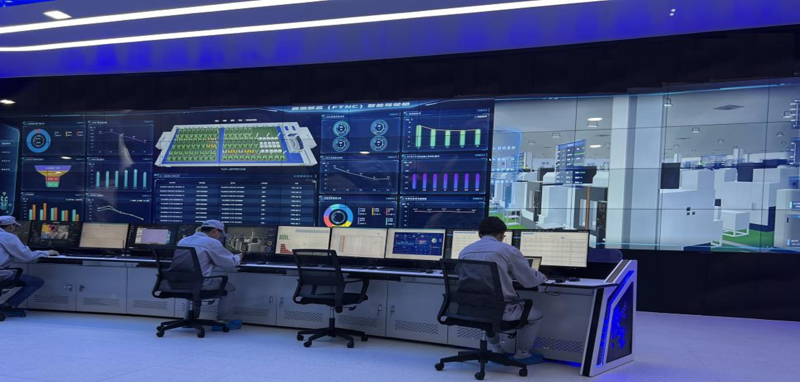
Central Control Room
