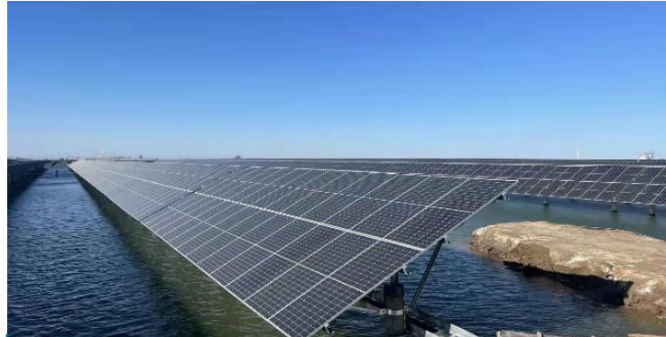
Shouguang, Shangdong, China 10MW Floating Solar Project
