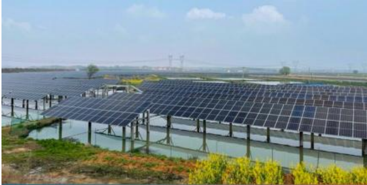
Xuancheng, Anhui, China 23MW Fishery Photovoltaic Project
