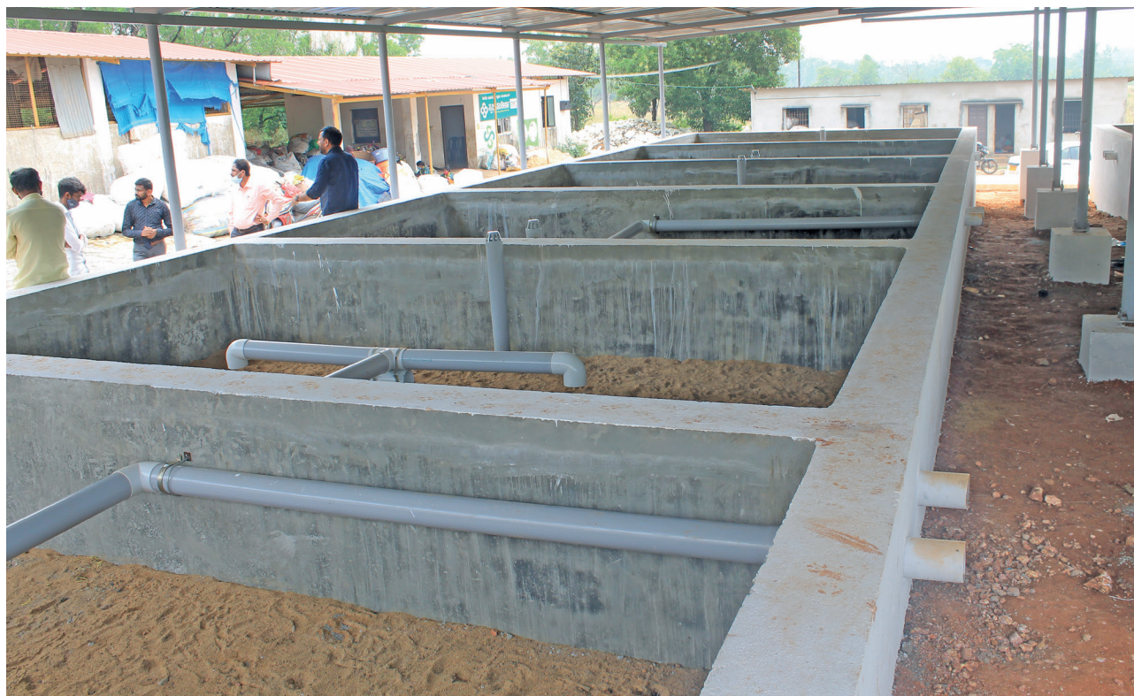
Karnataka's first rural faecal sludge treatment plant at 80 Badgabettu gram panchayat in Udipi district. The plant handles waste from six gram panchayats
