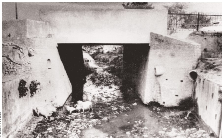
Noxious nitrates enter the groundwater through dirty waste-water drains
