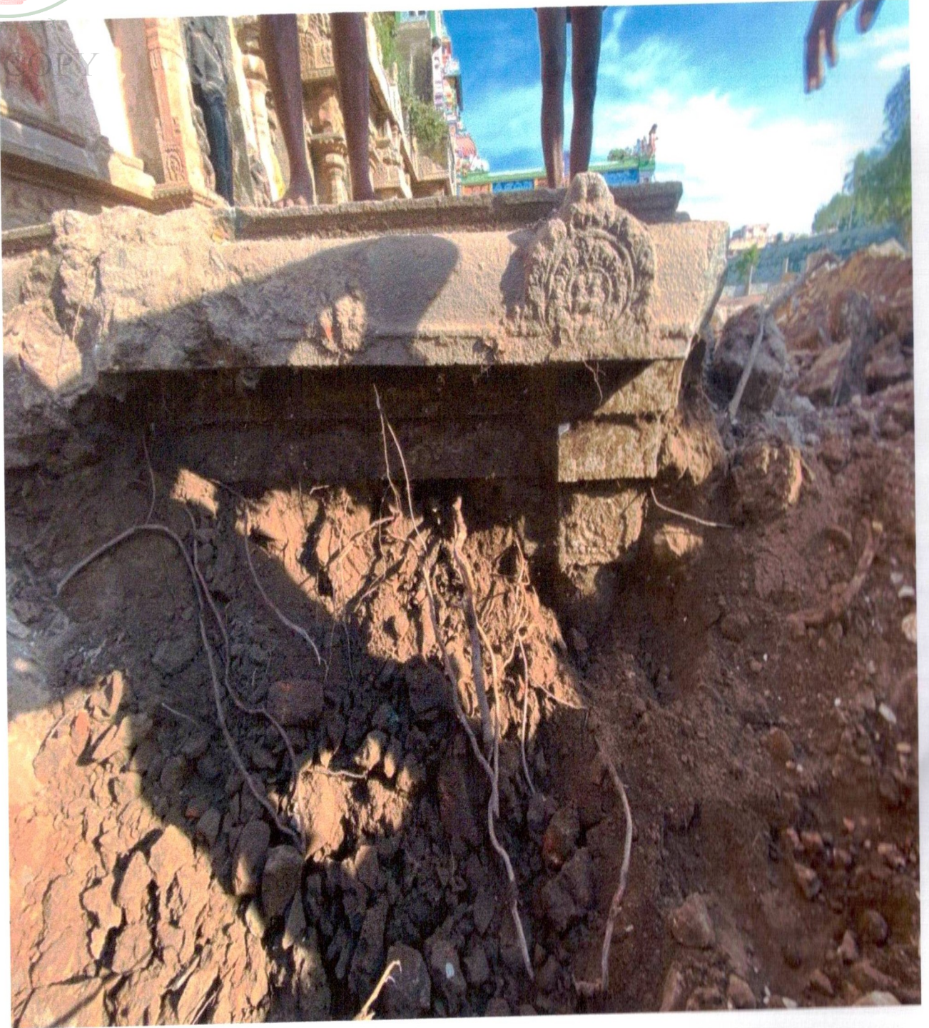
Dilapidated Bairavar Mandapam on West Entrance before restoration
