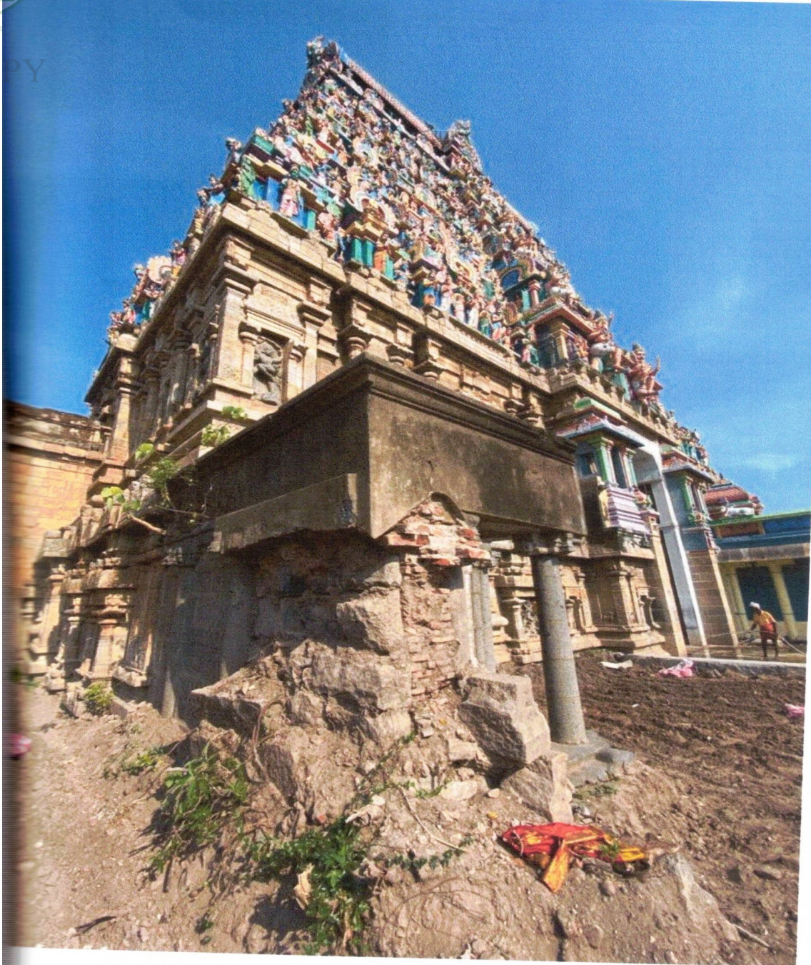
Dilapidated Bairavar Mandapam on West Entrance before restoration
